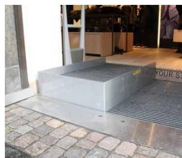
Lift on upper level, ready to enter/exit
